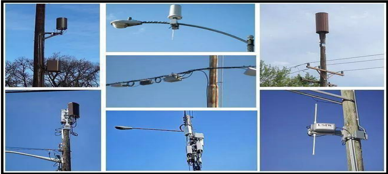
Examples of Small Wireless Communications Facilities
