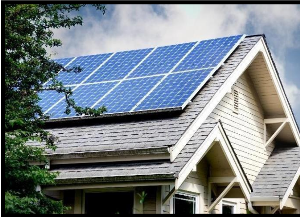
Roof solar panels
