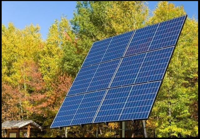
Stand-alone solar panels
